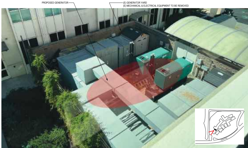
4 GENERATOR YARD BETWEEN MPK 10 & MPK 12
