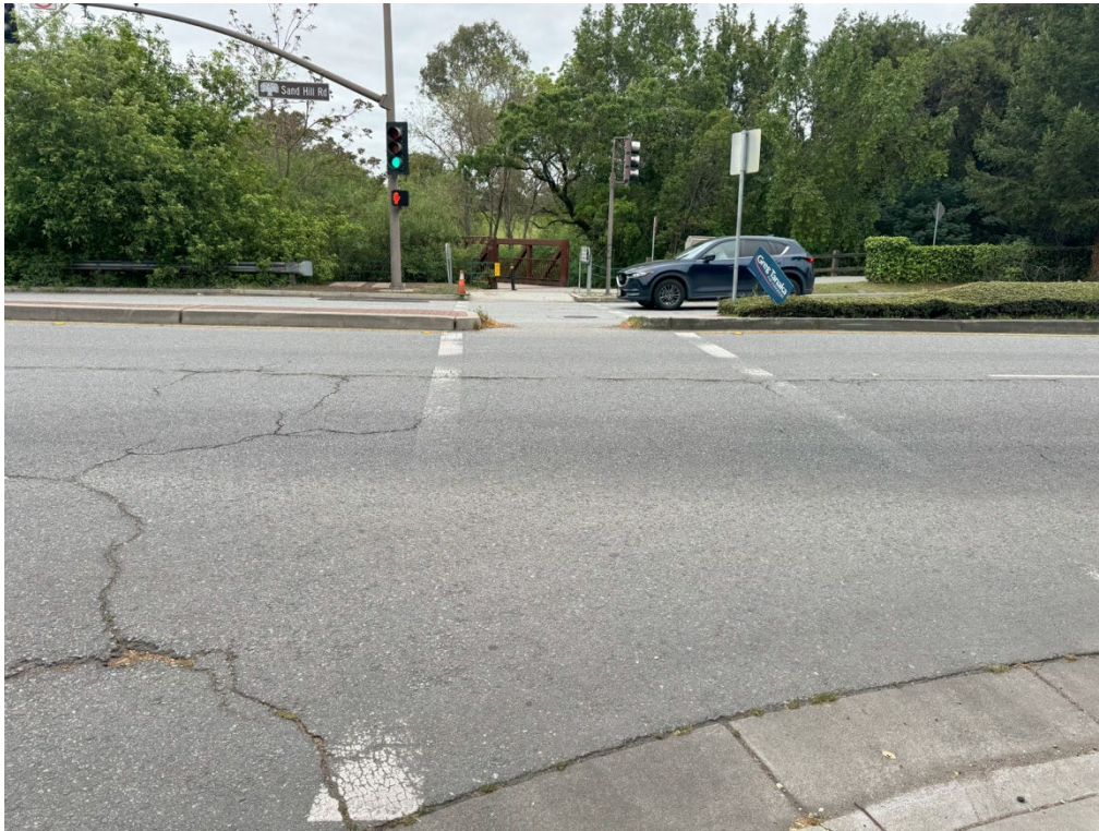
Figure 5-27: Worn Out Crosswalk Striping
