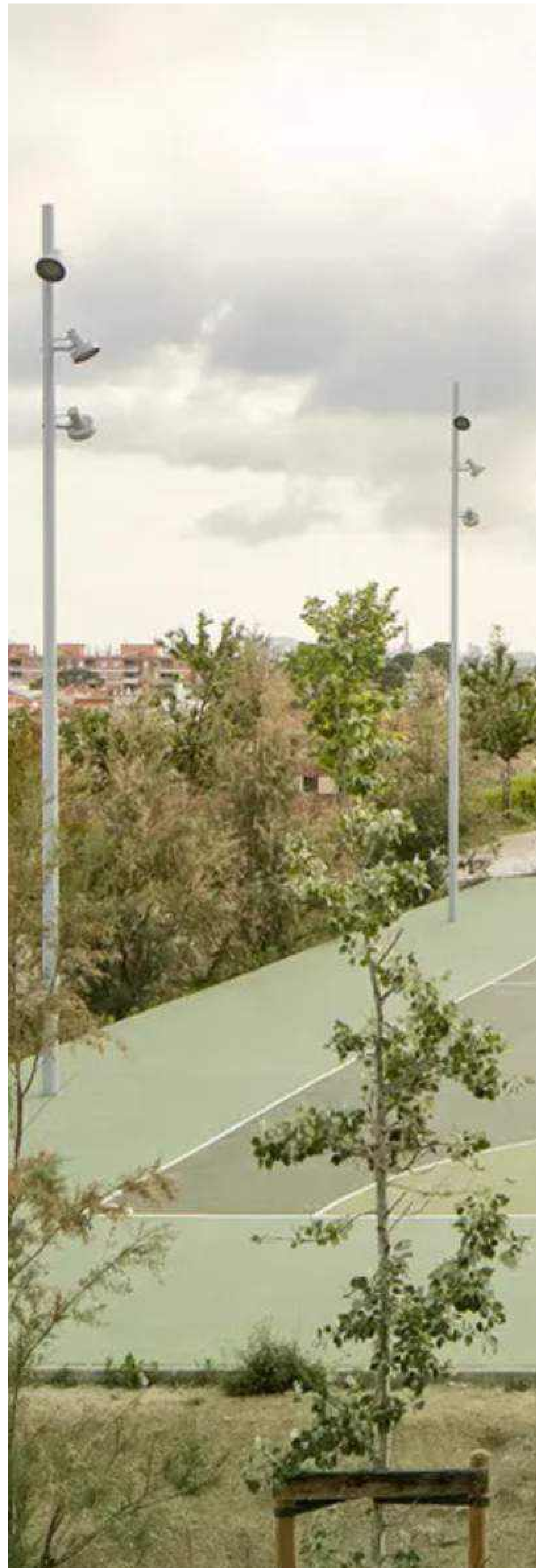
POLES WITH AIMMABLE FLOOD LIGHTS
