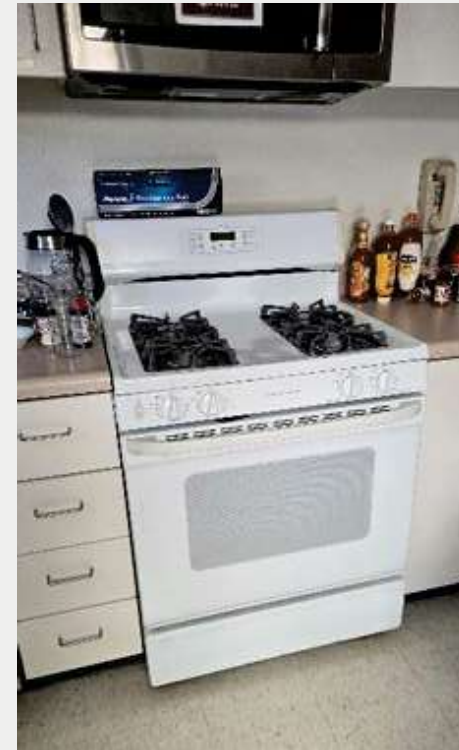
Gas stove in BHCDC
