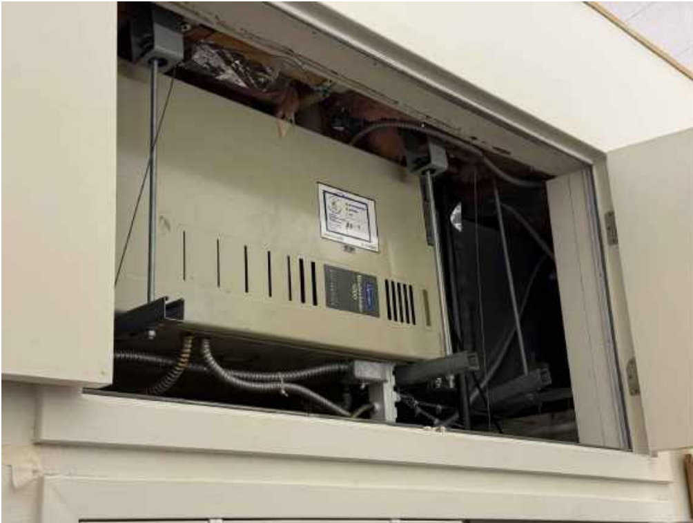
HVAC ACCESS PANEL
