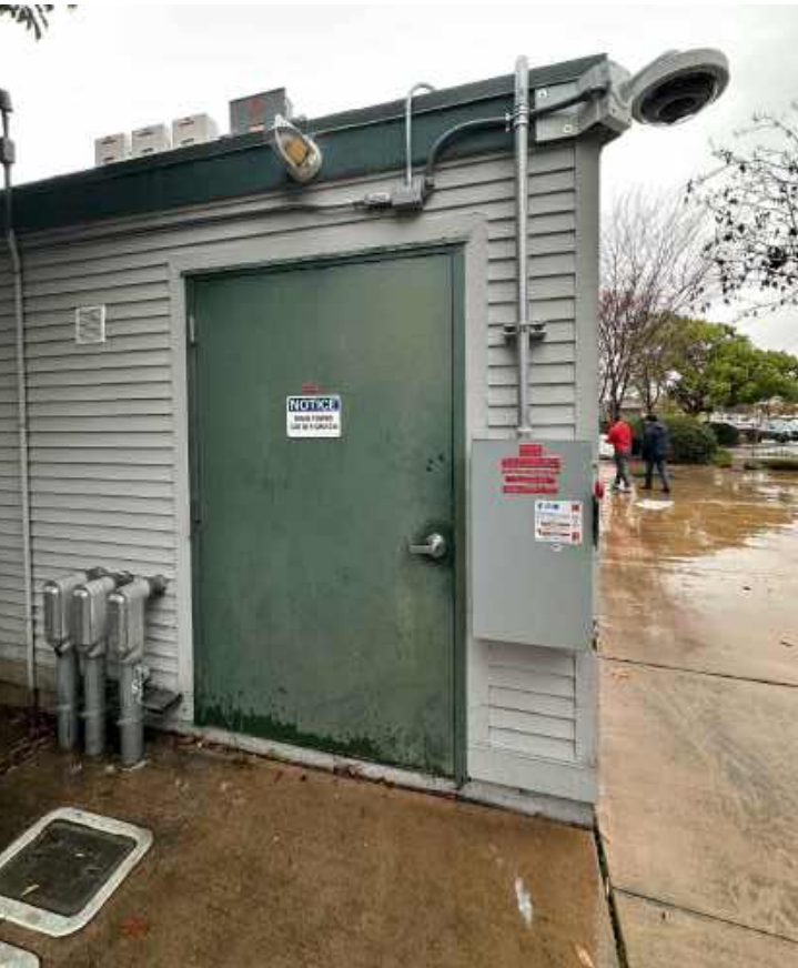
ELECTRICAL ROOM EXTERIOR
