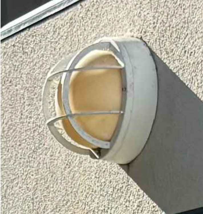
EXTERIOR WALL MOUNTED LIGHT
